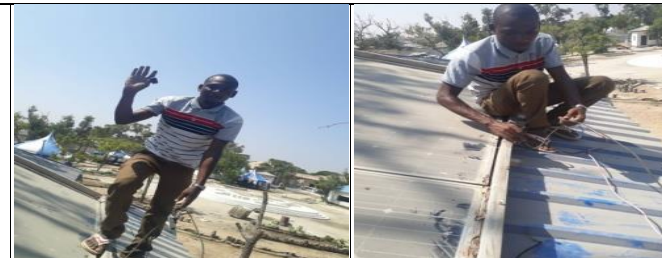
Basi team leader on top of the roof installing solar to a customer.
